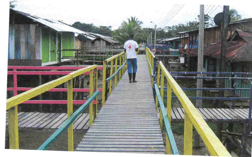
△ The IFRC assist in the construction of a new bridge using recycled materials.
