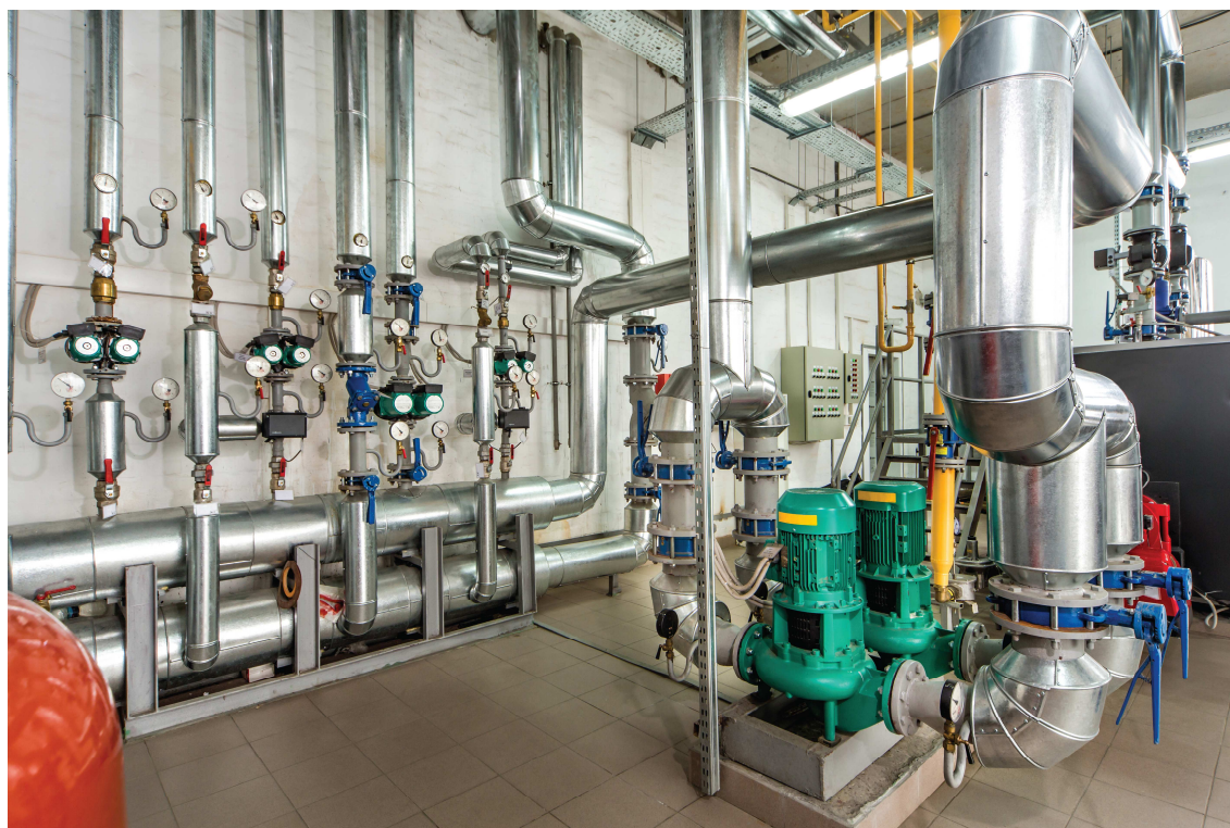
Figure 1 A heat pump at work
