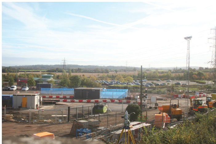
Photo. 1 The site of the new Oxford Parkway railway station – next to the Park and Ride
