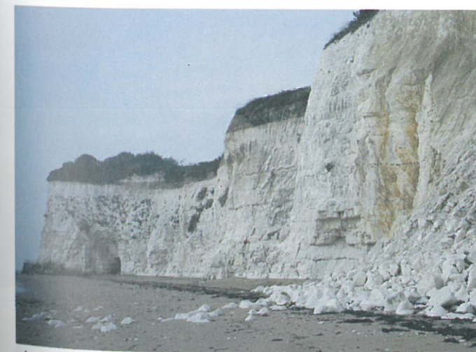
▲ Figure 2.22 Recent rockfall near Ramsgate in Kent affording temporary protection to that part of the cliff against further wave attack
