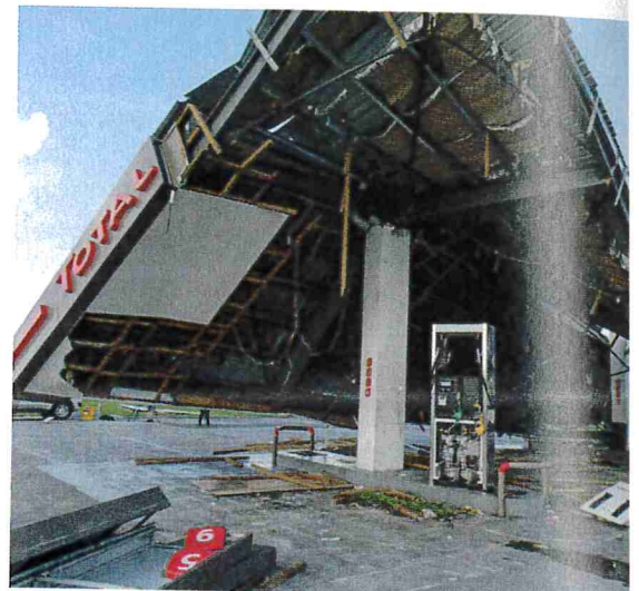
▲ Figure 5 Damaged caused by strong winds, Cyclone Winston, Fiji, 2016
