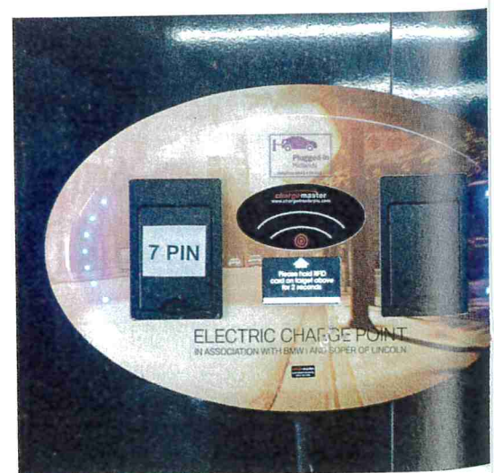
Figure 5 Charging points for HEVs, PHEVs and EVs are increasingly common, especially in city centre car parks
