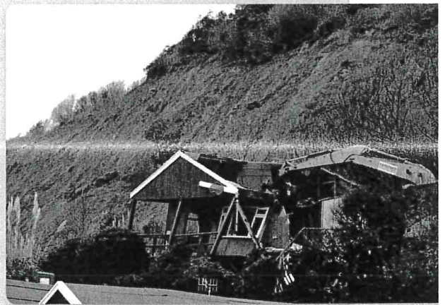
▲ Figure 3 One of seven holiday chalets that had to be demolished and removed from this location at Lyme Regis in 2014 following a series of landslips
