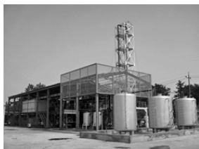
Plastics pyrolysis plant
