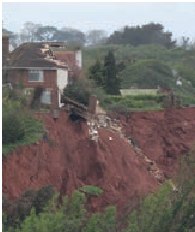
▲ A house destroyed by a landslide following heavy rain
