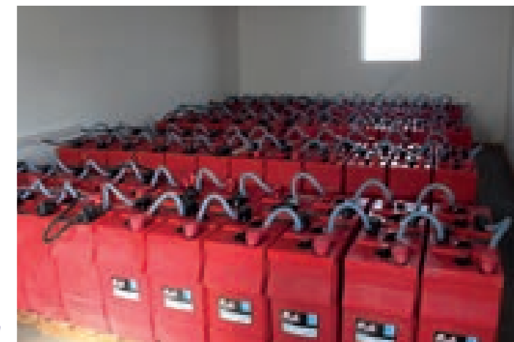
▶ A lead-acid battery storage system
