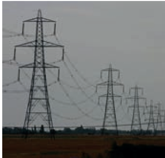
▲ Pylons and cables of the UK national grid
